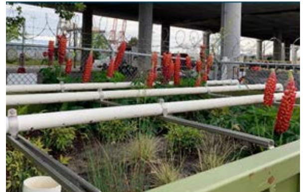
Figure 1. Plants and water distribution pipes at the top of the Horton Street maintenance yard Splash Boxx
